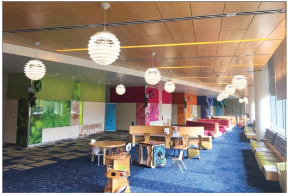
A look at Children's Hospital Colorado, where a 70 percent on energy savings occurred with the switch to LED.
